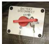
Battery Disconnect Switches
