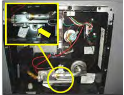
Water heater drain plug
