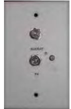
Antenna Power Supply
