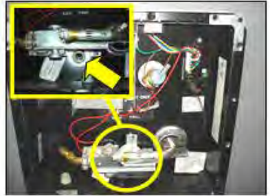
Water Heater Drain Plug
