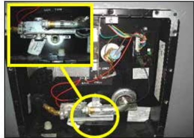
Fig 1: Water Heater Drain Plug
