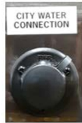
City Water Fill with City Water Connection Label
