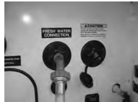
Black Tank Flush Inlet
