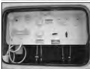
Fig. B Utility Center
