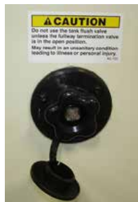
Tank Flush Inlet
