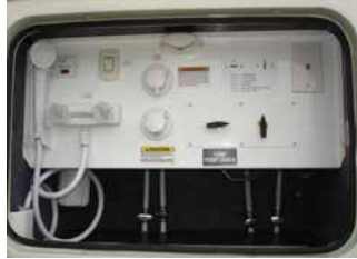
Fig. B - Utility Center
