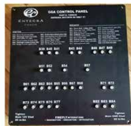
GFCI Breaker Panel
