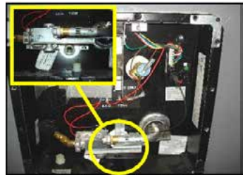
Fig 1: Water Heater Drain Plug
