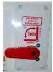
Water Heater Bypass Valve
