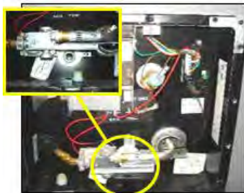
Fig 1: Water Heater Drain Plug
