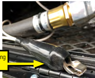
Grounding Clip Inside Fuel Station
