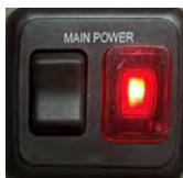
Battery Disconnect Switch
