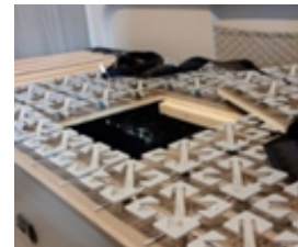
Water Heater Bypass Access
