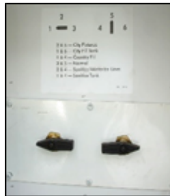
Fig.A - Water Valve Controls
