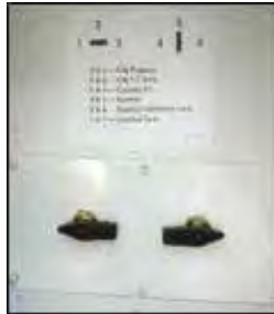
Fig.A - Water Valve Controls
