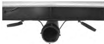
Black/Grey tank drain & valves
