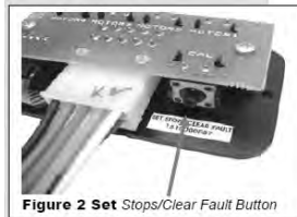
Figure 2 Set Stops/Clear Fault Button
