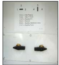
Fig. A - Water Valve Controls
