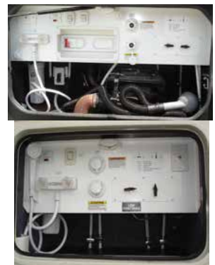
Fig. B - Utility Center
